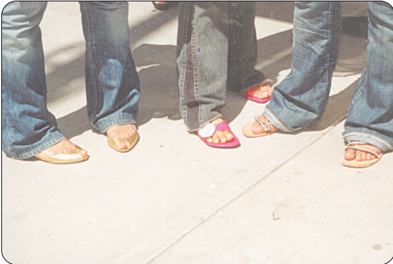
An example of the existing concrete sidewalks the City Manager would like to see replaced with granite.
